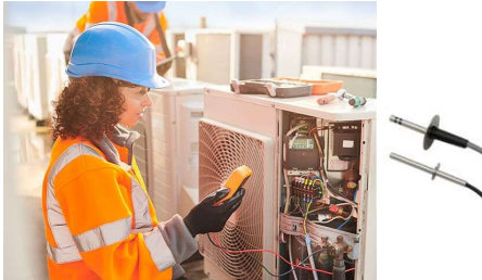
Heat Pumps (HVAC)
