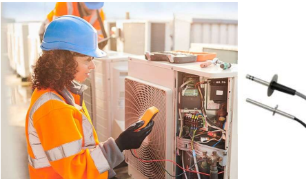
Heat Pumps (HVAC)
