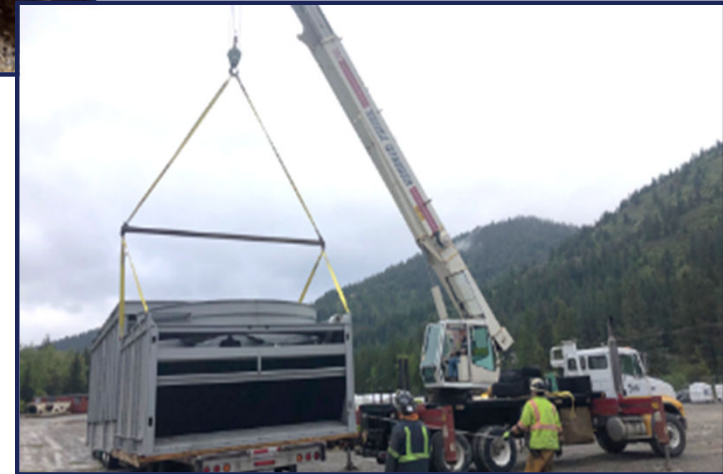
Surface Cooling Project
