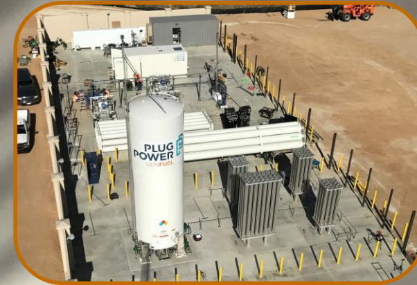
Skid: Modular Hydrogen System
