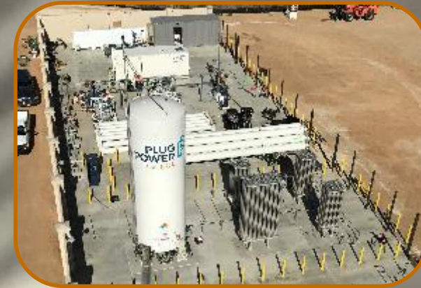
Skid: Modular Hydrogen System
