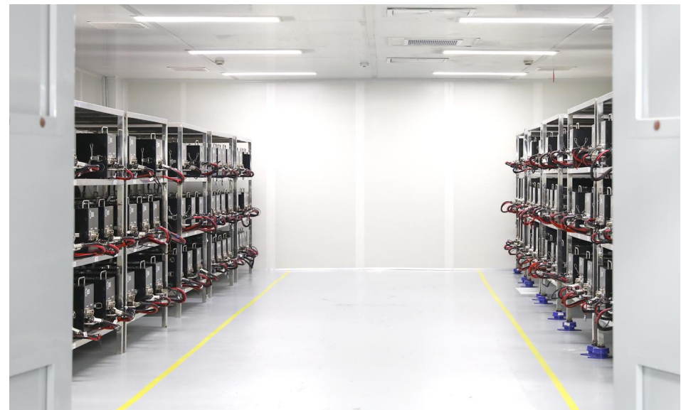
Test bunker for automotive Li-Metal cells
